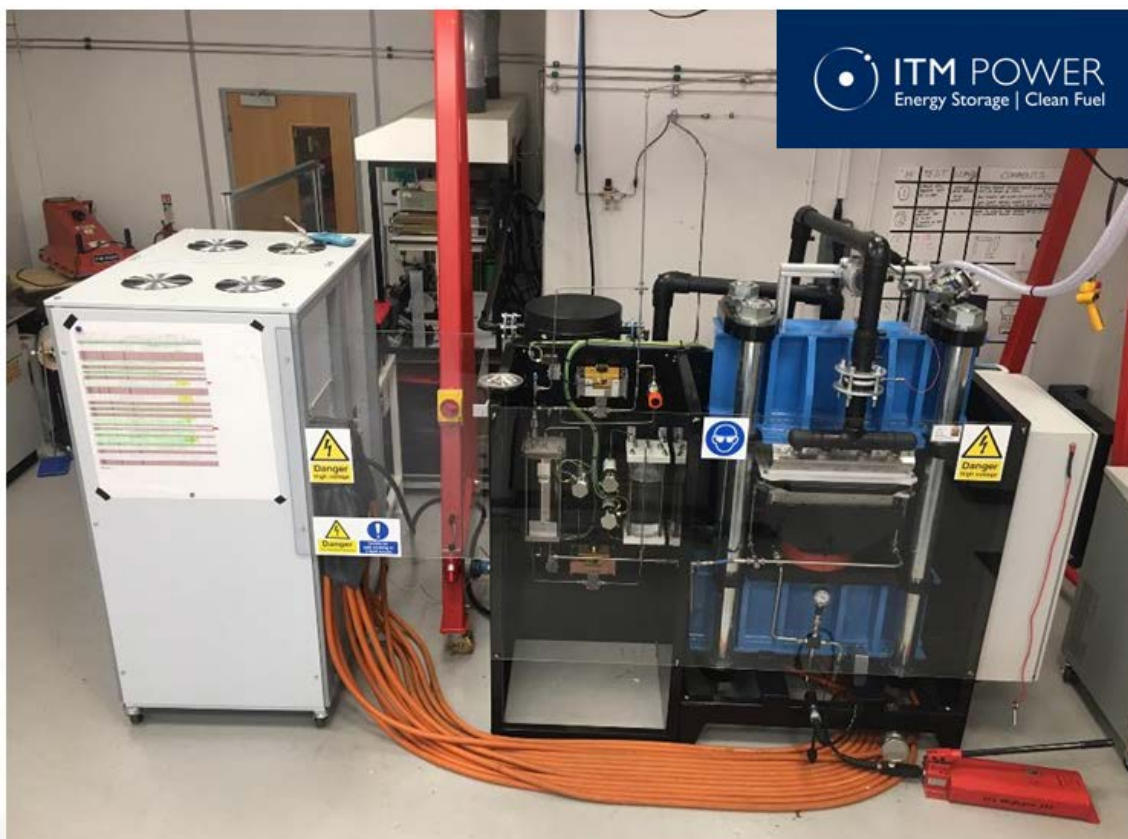
Figure 1 - as build stack test stand
