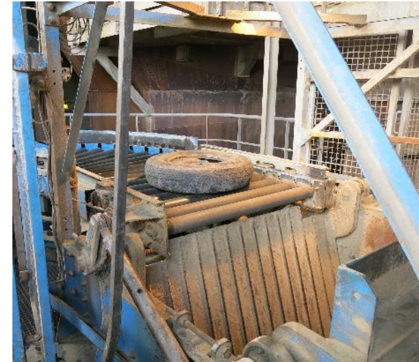
Calciner fuel feed
