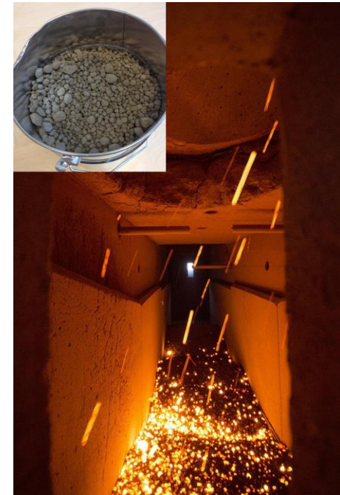
Hot commissioning of the oxyfuel clinker cooler and first oxyfuel clinker samples
