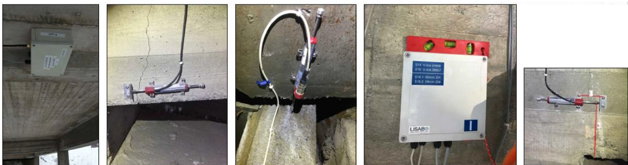
Figure 78: Installed sensors, Foto: NPRA
