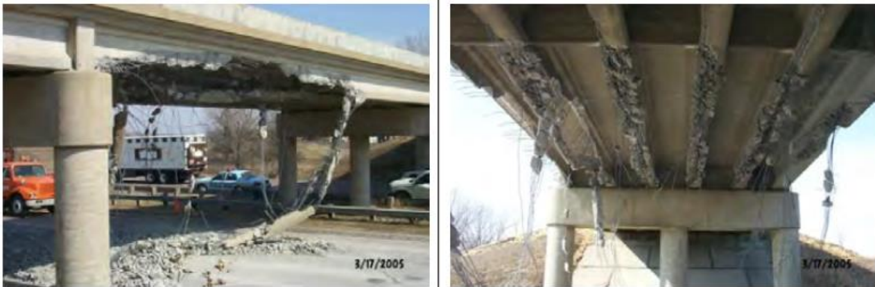
Figure 2. Damages due to vehicle impact: Vehicle impact to Sgt. Bluff bridge in Iowa, March 17, 2005 (Harries et al., 2012)
