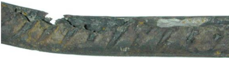
Figure 12. Pitting corrosion in reinforcement caused by chlorides. Reinforcement extracted from a quay in northern Norway.
