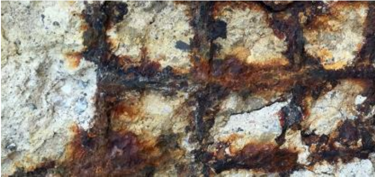
Figure 7. Corrosion caused by carbonation (Täljsten et al., n.d.)
