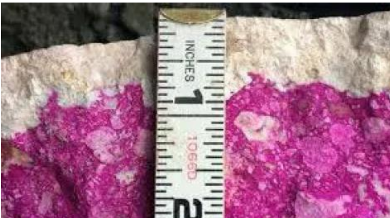
Figure 8. Application of phenolphthalein on a recently exposed concrete surface, an uncoloured area indicates carbonation (www.structuralguide.com)
