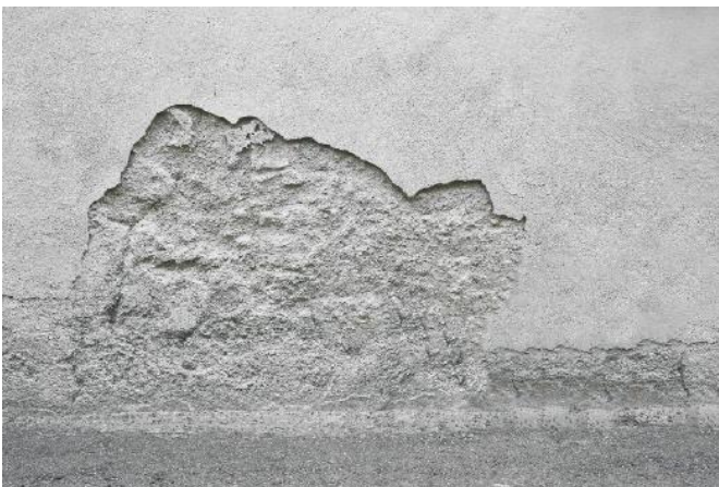
Figure 4. Example of frost damage in concrete that has caused delamination on the surface. www.fritzpak.com
