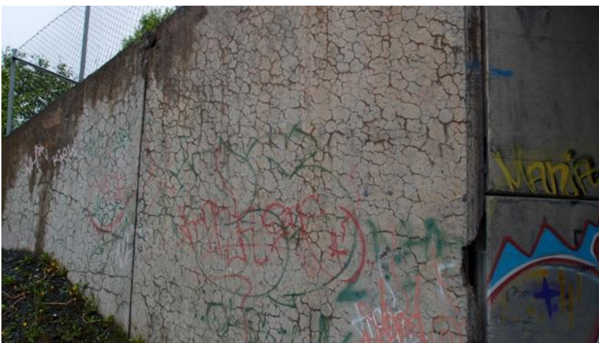
Figure 4-4: Characteristic map cracking on a surface due to ASR
