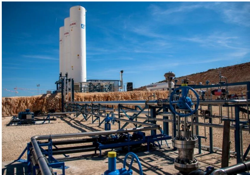
Hontomín site, showing the CO 2 pipeline from the storage tanks to the injection well
