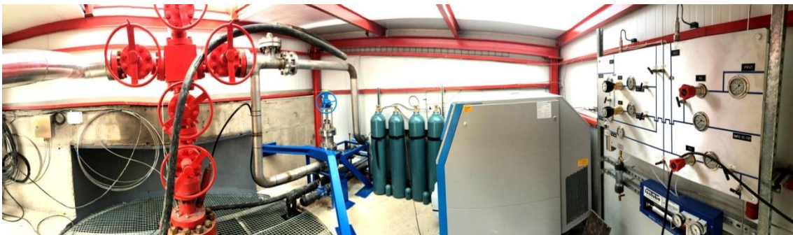
CO 2 Injection well (H-1, left) and U-tube system (control board, right) at Hontomín. The CO 2 pipeline leading to the well head is clearly visible in the centre of the image.
