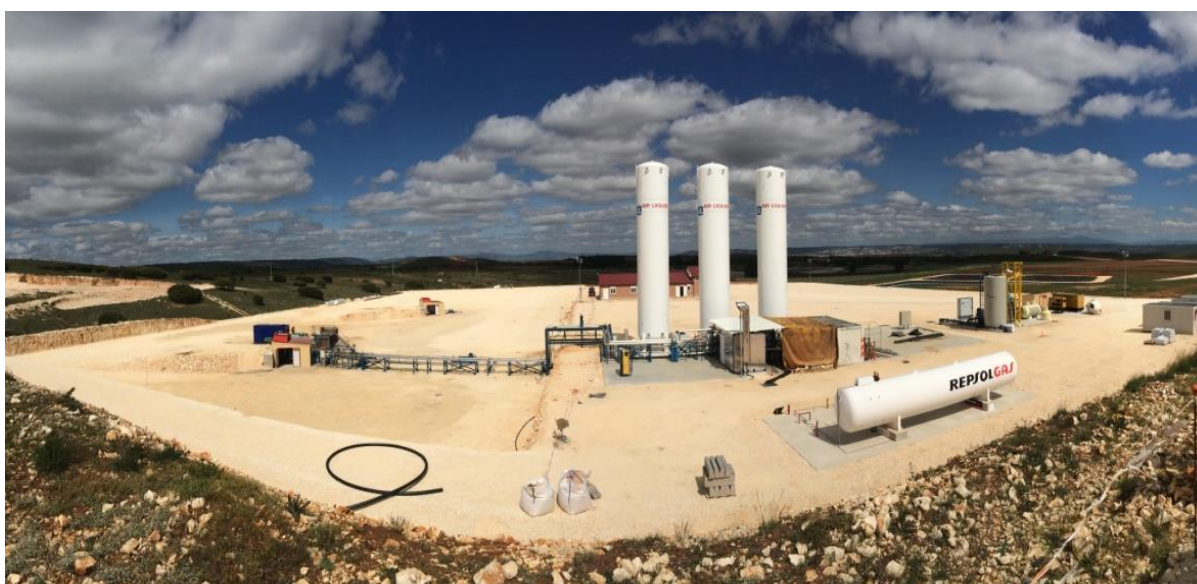
Panoramic view of the Hontomín site, showing the CO 2 storage tanks (just right of centre), the injection well (inside the small building on the left) and water storage reservoirs (at the far right).
