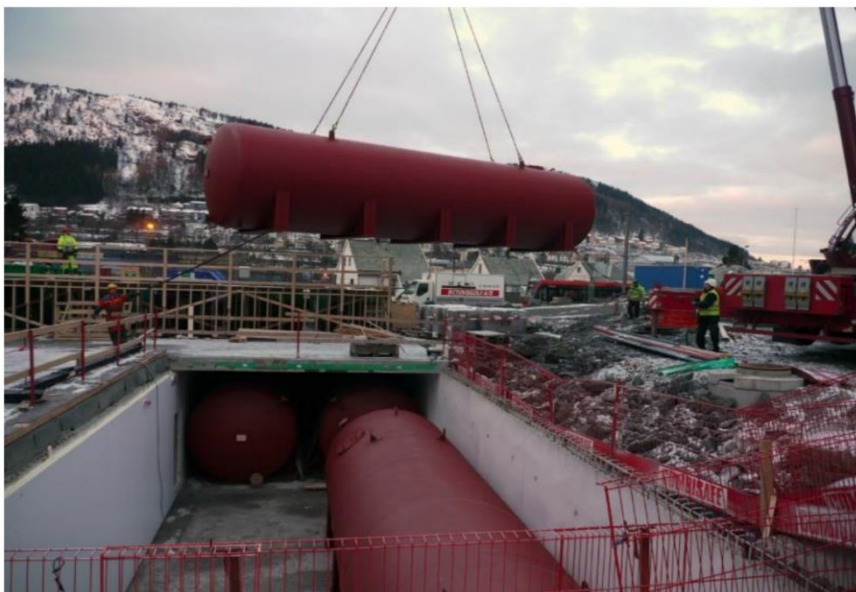
Figure 3 – PCM cold storage tanks of University College Bergen (Dar2014)
