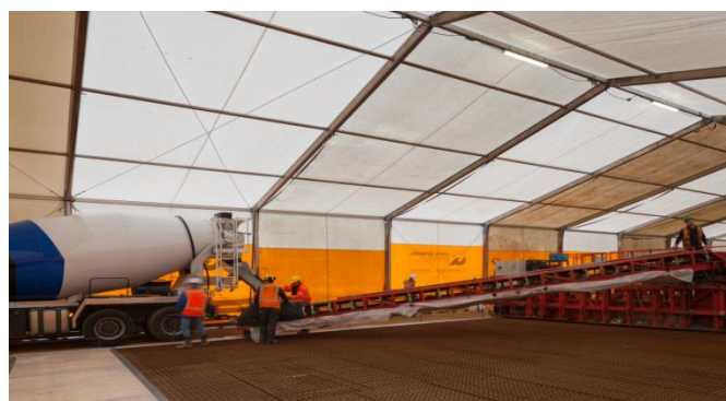
Figure 2: 100 m of bridge slab could be paved in one day. (Photo: Bart van Hoek)
