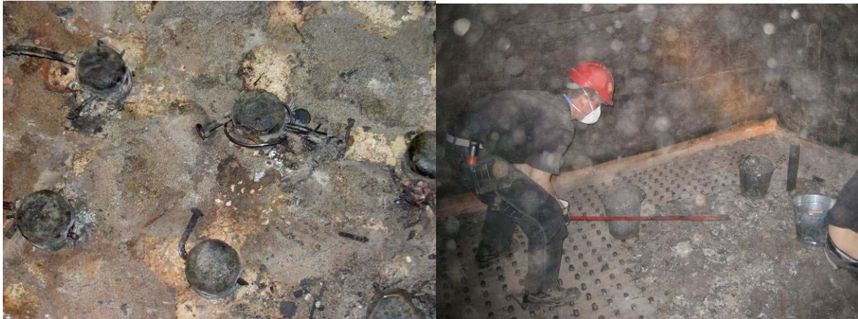
Figure 1.5. Fluidized bed plugged nozzles (left) and manual cleaning (right) before retrofitting.
