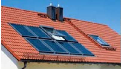
Solar thermal - decentralized
