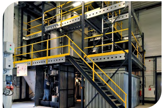
BTG's pilot plant for pyrolysis of biomass (200 kg/h)
