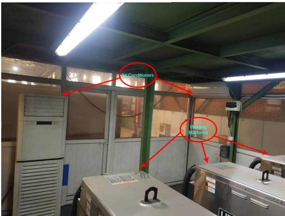
Figure 66:Welding Machines in a Closed Room at Noksel
