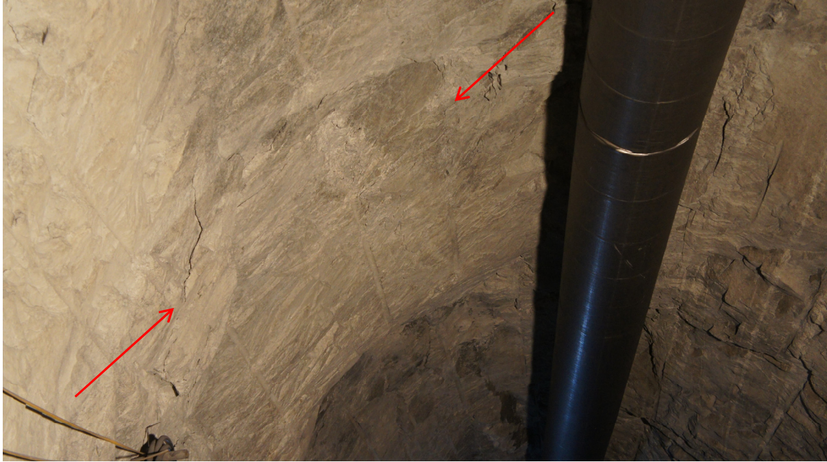
Fig. 7. High stress causing rock burst in some section of the headrace tunnel.
