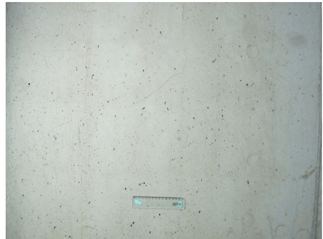
Figure 4b: Picture of pores on a concrete surface.
