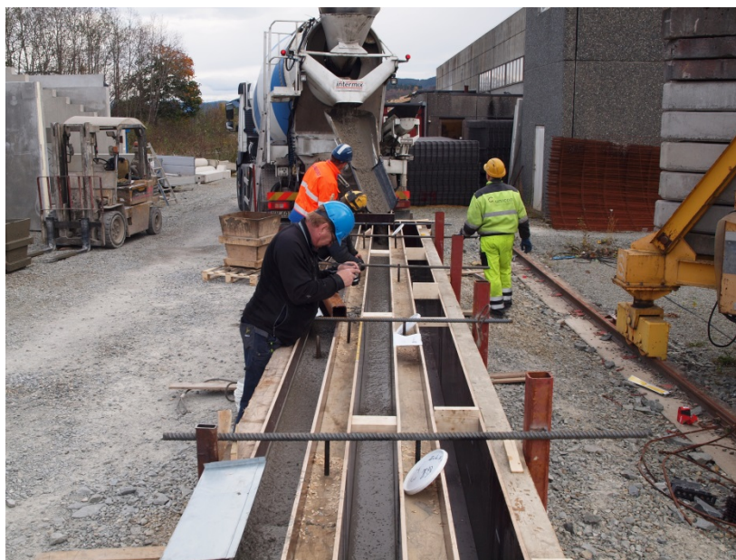
Figure 3: In search for a test method and criteria to evaluate the stability of SCC Picture of the field test – flow of concrete over a longer distance might provoke the concrete segregate resulting in an inhomogeneous concrete element with inferior structural and durable properties
