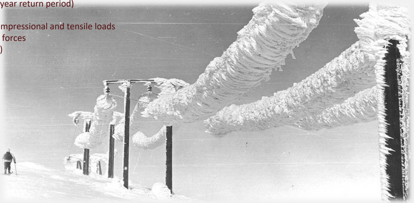
«Record» in icing on power line (22 kV), ca. 1.5 m ice that constituted ca. 300 kg/m line Picture from Lønahorgi, 1961 (Olav Wist)
