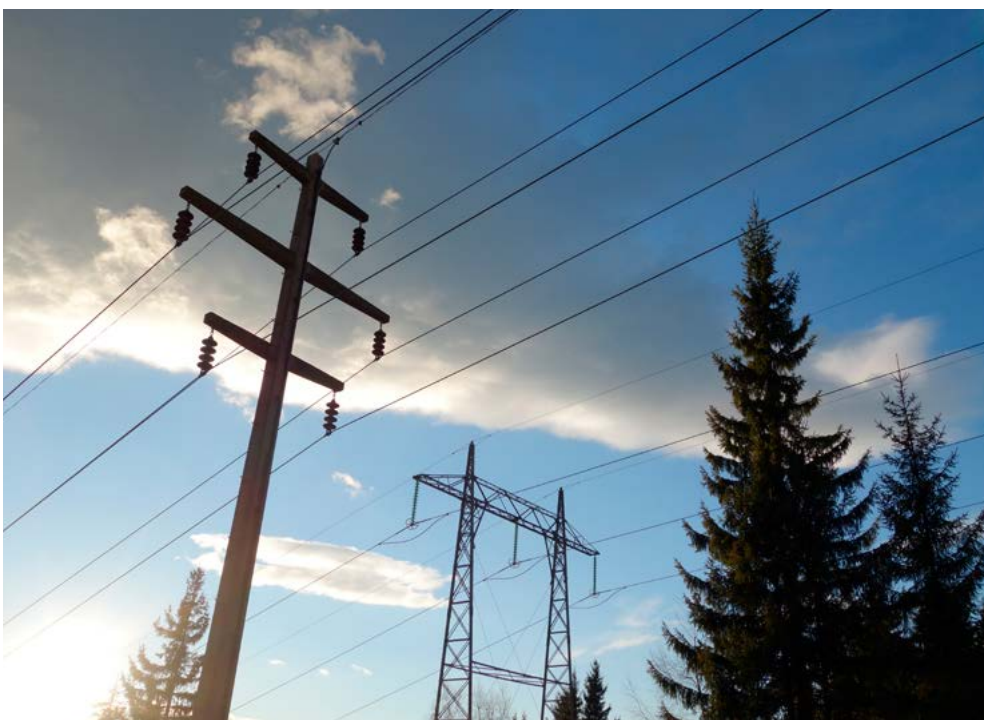
Conflicts often arise when new power lines are planned and constructed. Studies carried out in HydroBalance show that disagreements can be avoided or significantly reduced Photo: Øystein Aas
