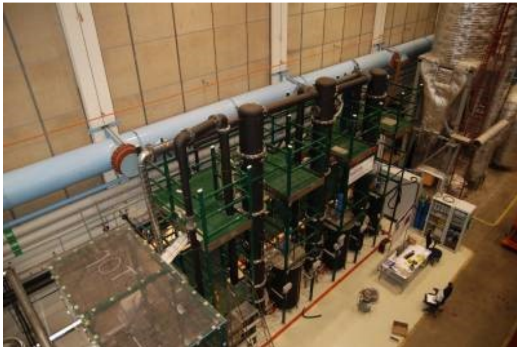
CAP pilot plant used for CEMCAP tests (photo by GE Power Sweden)
