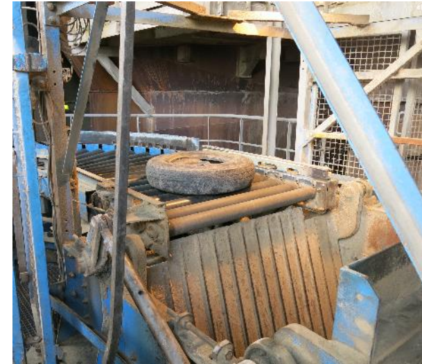
Calciner fuel feed
